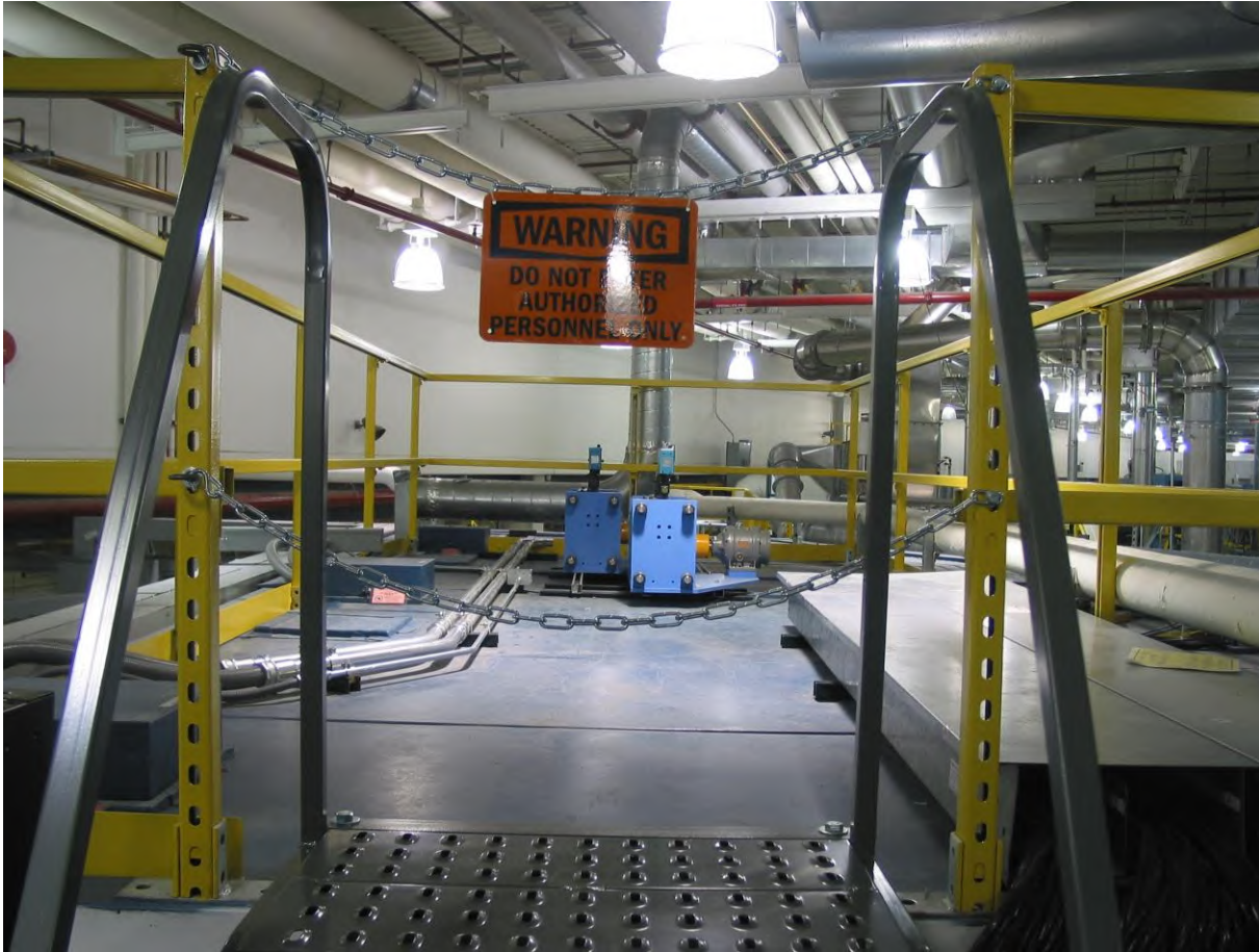
Figure 4. Two 200 MPa hydraulic pumps for controlling the differential rams in DDIA-30. These pumps have been mounted on the roof top of 13-ID-D. Hand rails, steps, and warning signs have been installed. Hydraulic lines into the hutch will be installed in May, 2010. Note that this location is restricted to authorized personnel only.
